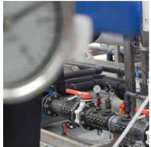
Sea water desalination plant SPAIN
