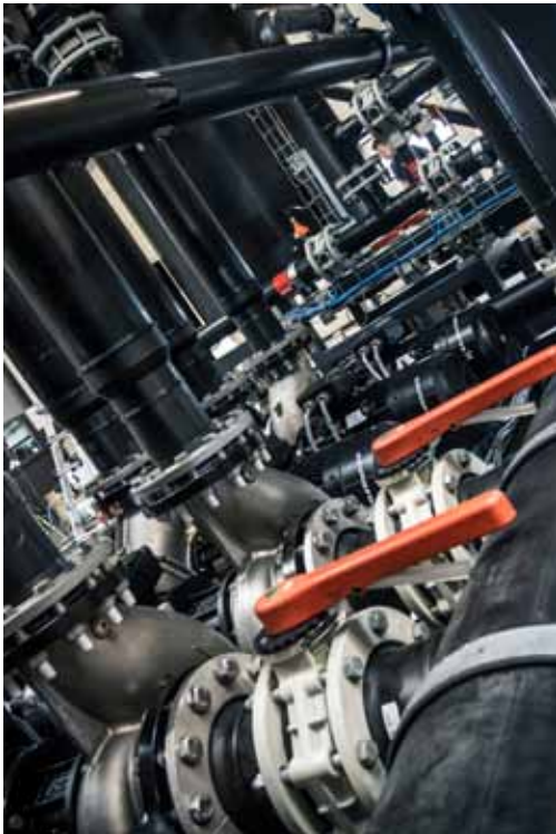
Oil plant - filtration VENEZUELA
